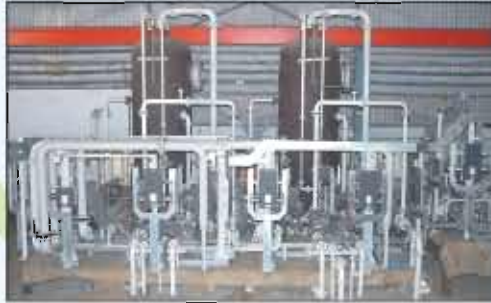
Mix Bed & Dosing Skid (CPU)
