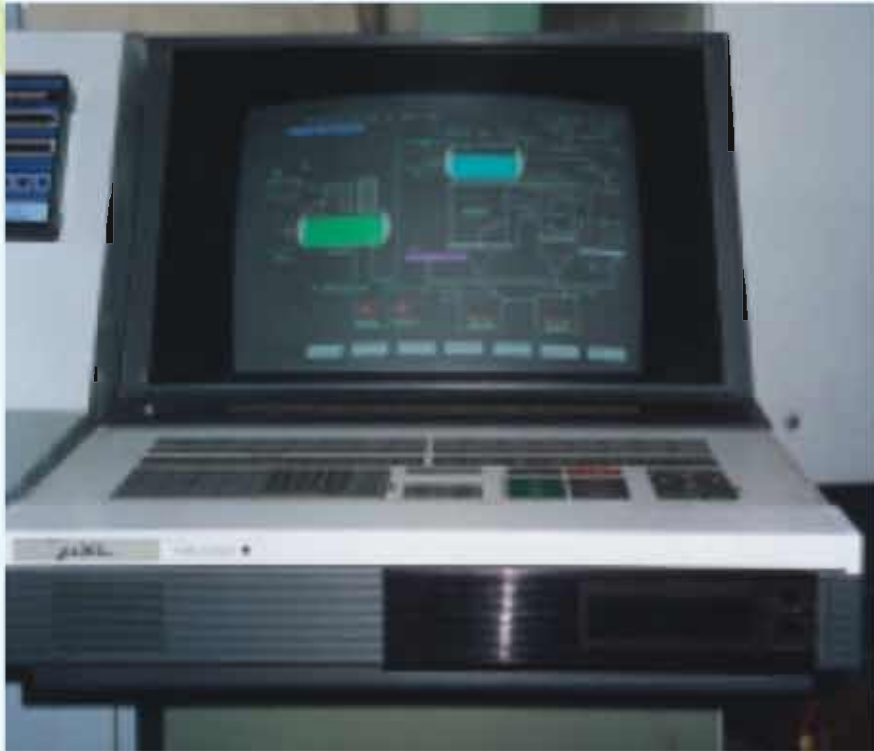
Insert of DCS Control System for Incinerator Plant
