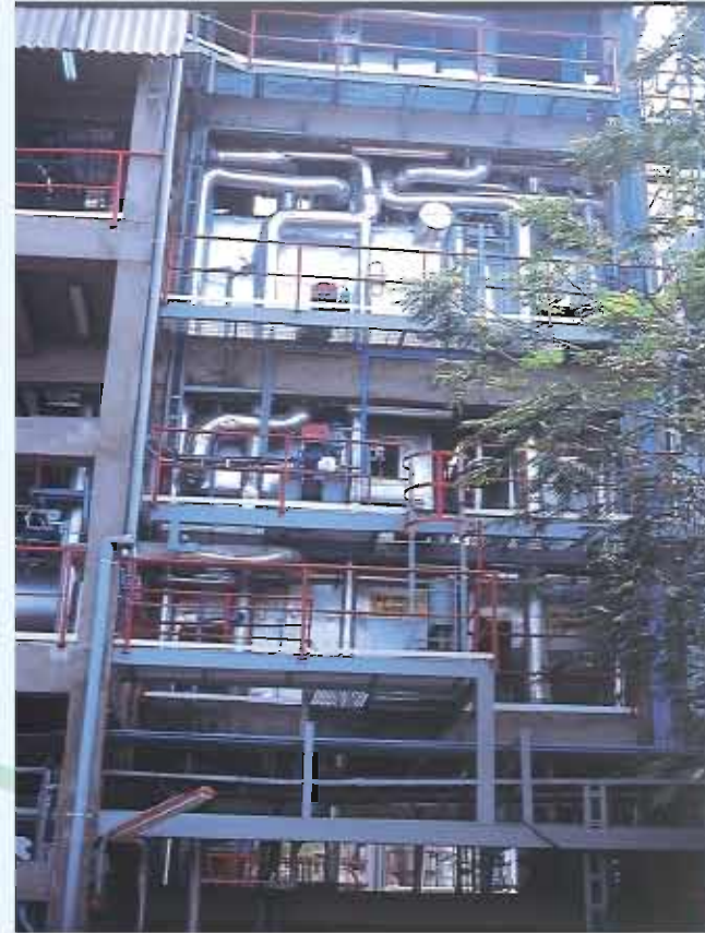
View of Waste Heat Recovery Boiler
