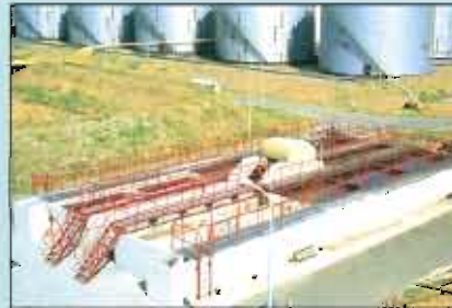
Oil-Water Separator (CPI)
