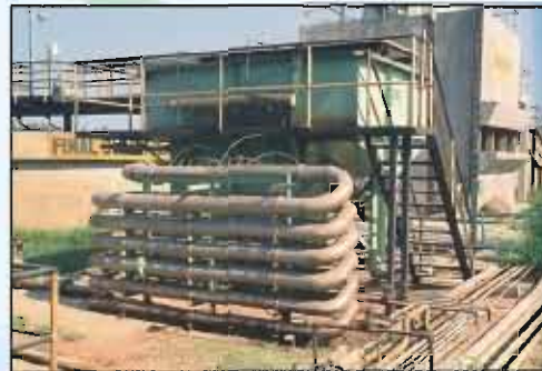
Coiled Pipe Flocculator
