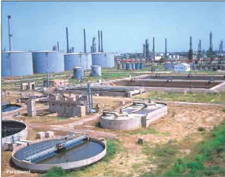
Indian Oil Corporation Ltd, Vadodara - 1600 m 3 /hr Capacity
