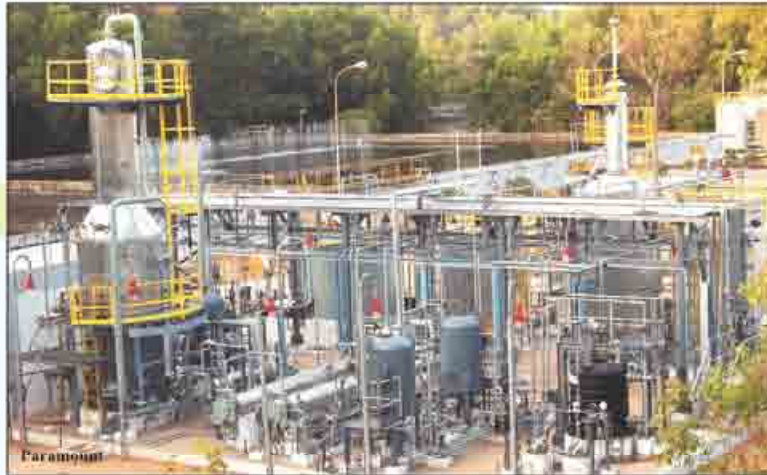
MRPL, Mangalore Wet Air Oxidation Plant 5 m 3 /hr
