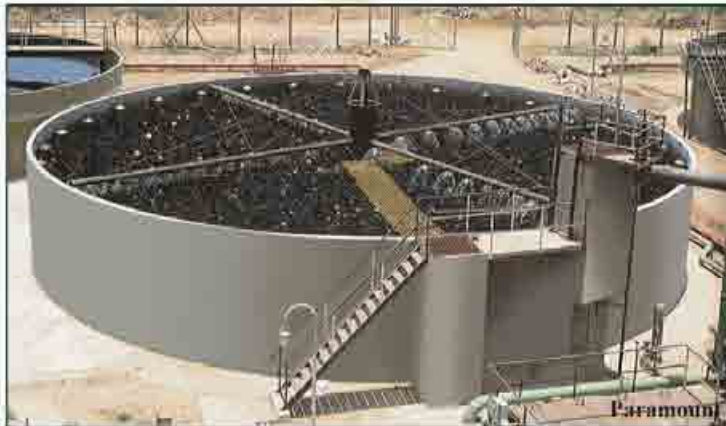
Plastic Media Bio-Tower Alembic Limited, Gujarat
