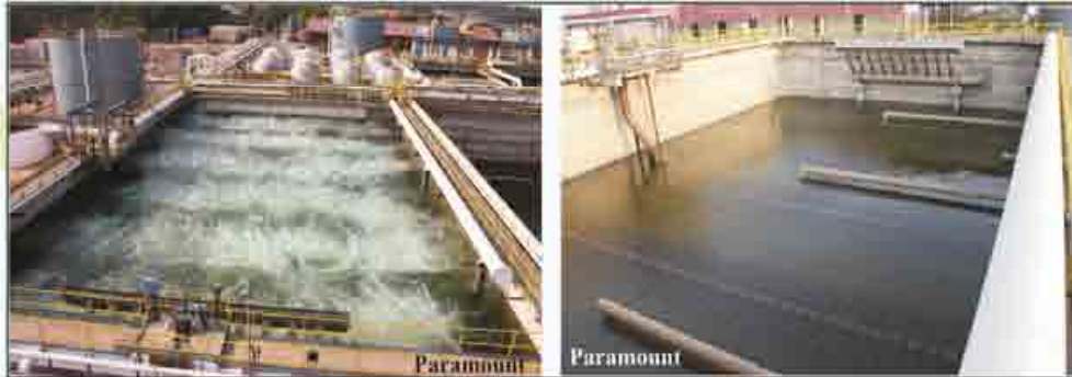
Sequential Batch Reactor (SBR) Mangalore Refinery & Petrochemicals Ltd., Mangalore(MRPL)
