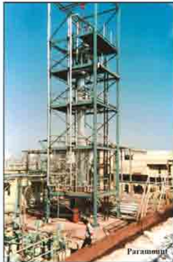
ONGC, Hazira 1 m 3 /hr Wet Air Oxidation Plant
