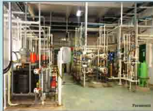
Skid Mounted Recycle System
