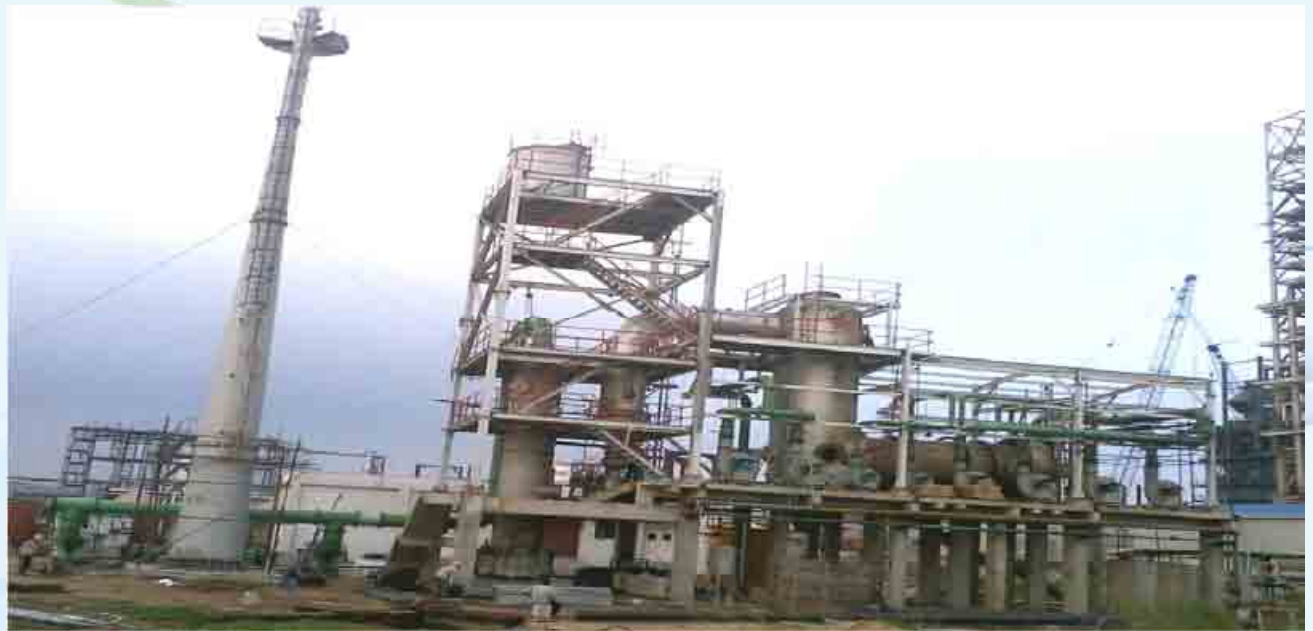
Incinerator at IOCL, Paradeep for Solid Waste (Oily Sludge and Spent Carbon)
