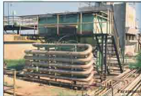
Coiled Pipe Flocculator
