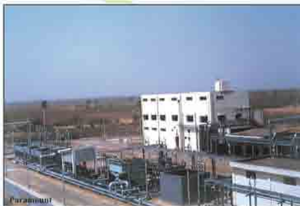
Water Re-injection Plant & ETP for ONGC, Mehsana
