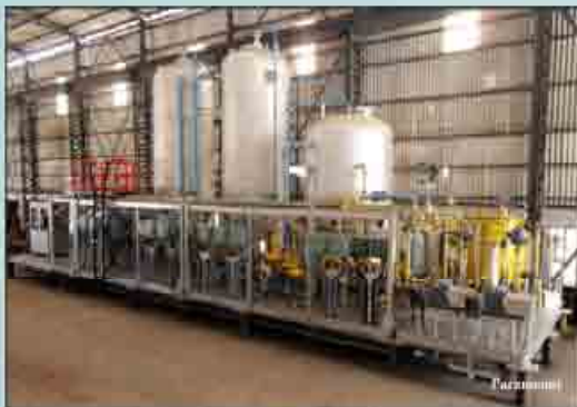
Skid Mounted CPU System
