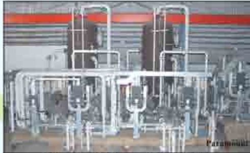
Mix Bed & Dosing Skid (CPU)
