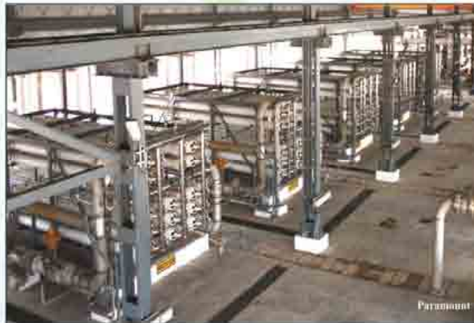
RO Skids at M/s. Mangalore Refinery & Petrochemicals Ltd.
