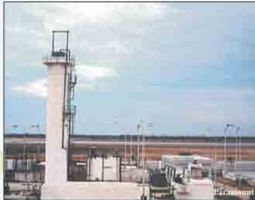
Anaerobic Upflow Fluidised Bed Reactor (UFB) Orchid Pharma & Chemicals Ltd, Chennai
