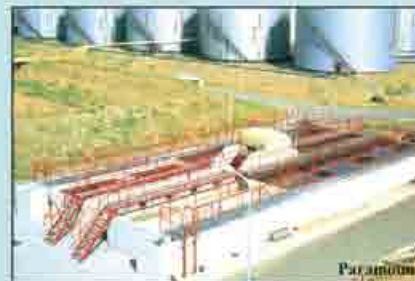
Oil-Water Separator (CPI)
