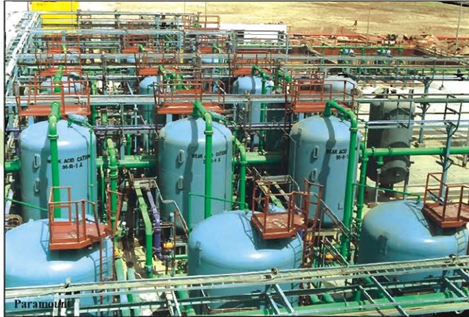
D. M. Plant 600 m 3 /hr, 4 chains of 150 m 3 /hr
