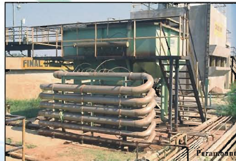
Coiled Pipe Flocculator
