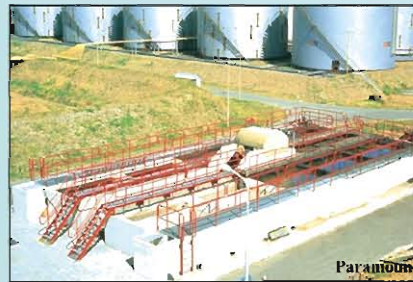
Oil-Water Separator (CPI)
