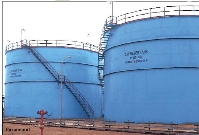
D. M. Water Storage Tanks
