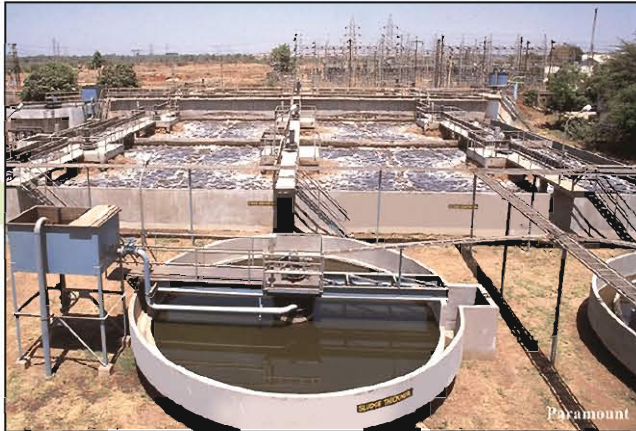
15 MLD CETP at Thane Belapur TTC Industrial Area
