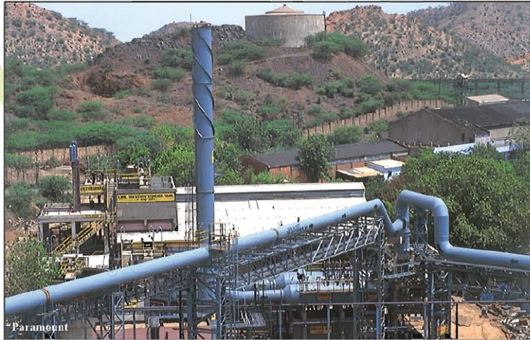
Large FGD unit at Hindustan Copper
