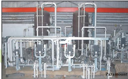
Mix Bed & Dosing Skid (CPU)
