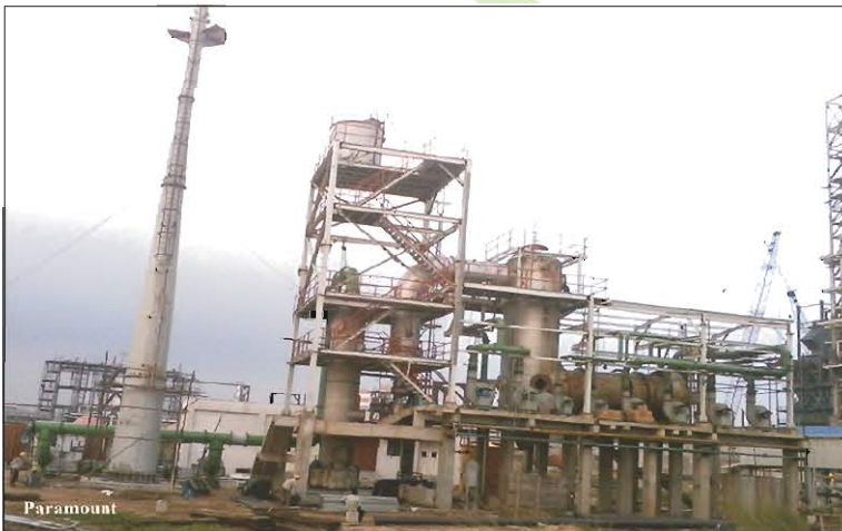
2000 T/Yr Incinerator at Indian Oil Corporation Ltd., Paradip
