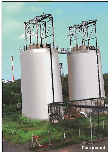
Upflow Anaerobic Sludge Blanket Reactor (UASB) Alembic Limited, Gujarat
