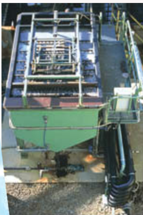
CPF-TPF for a coke oven effluent of steel plant
