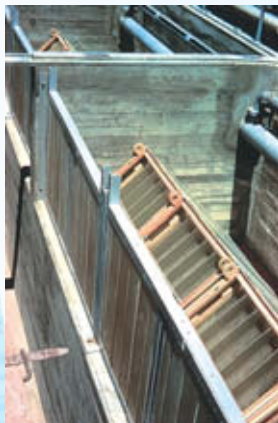
TPI internals in concrete tank
