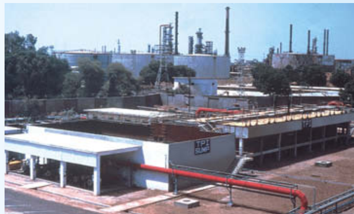
A large TPI in concrete basin (Cap. 1500m 3 /hr) at 12.5MMTPA refinery
