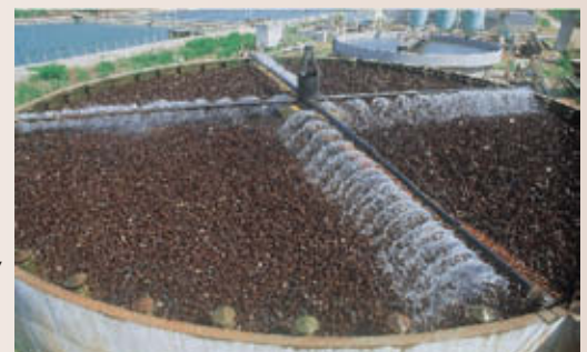
A view of Bio-Tower for a Refinery
