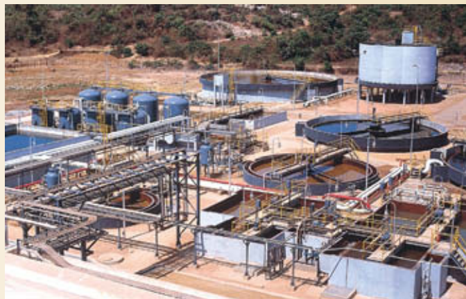
A view of a DAF at a Refinery
