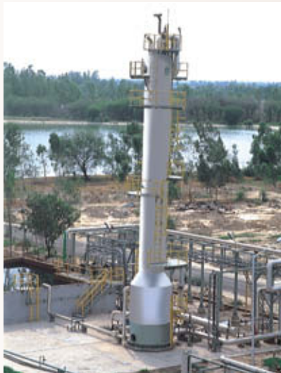
Ammonia steam strippers at a Fertilizer Complex
