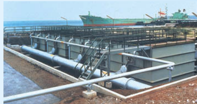
Battery of TPI's for ballast water
