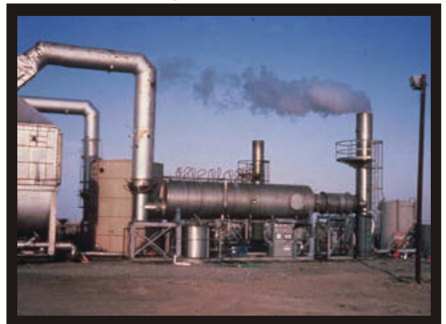
SO 2 Scrubbers for utility boilers burning high sulphur fuel
