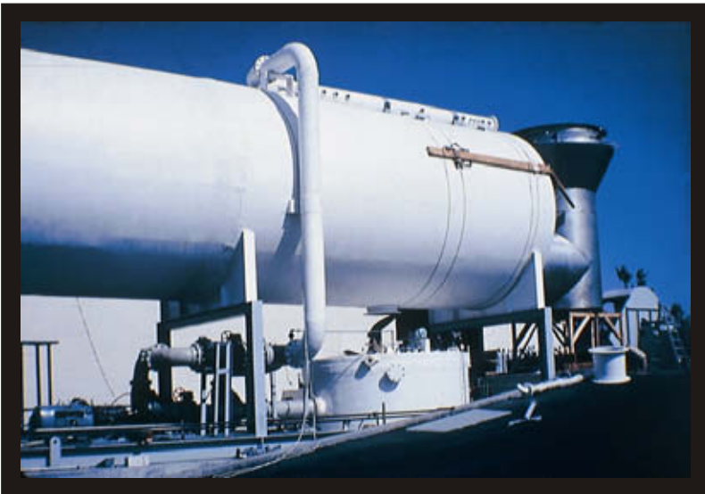
View of a large FGD unit with FRP Scrubber
