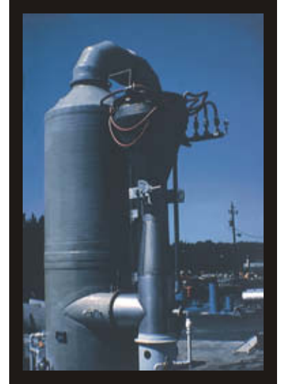
Incinerator Scrubber with Venturi and Packed Tower
