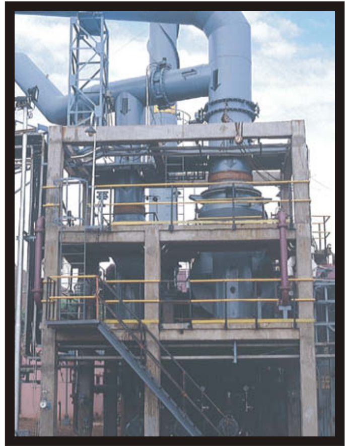
View of Quench for SO 2 Scrubbers
