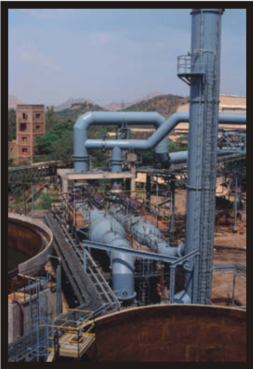
FGD with Double Alkali Process at a Copper Smelter
