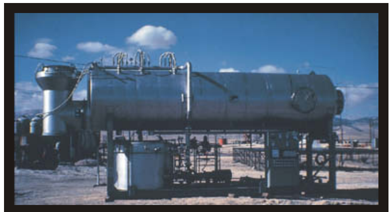
FGD for a heavy Oil Fired Steam Generator
