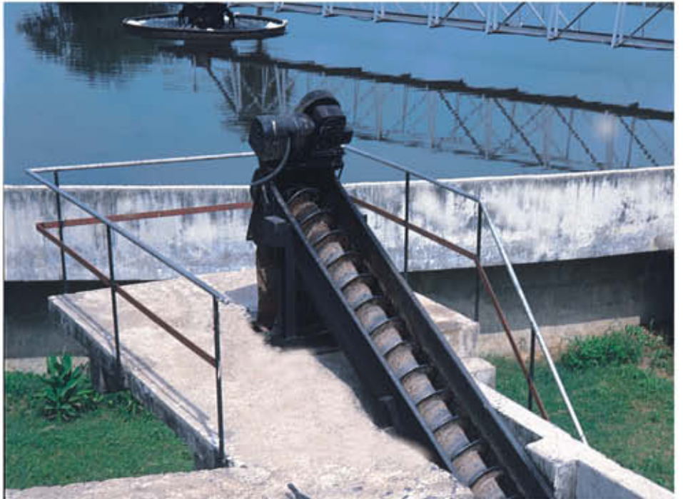
Grit separator and primary settling tank at a Municipal sewage treatment plant
