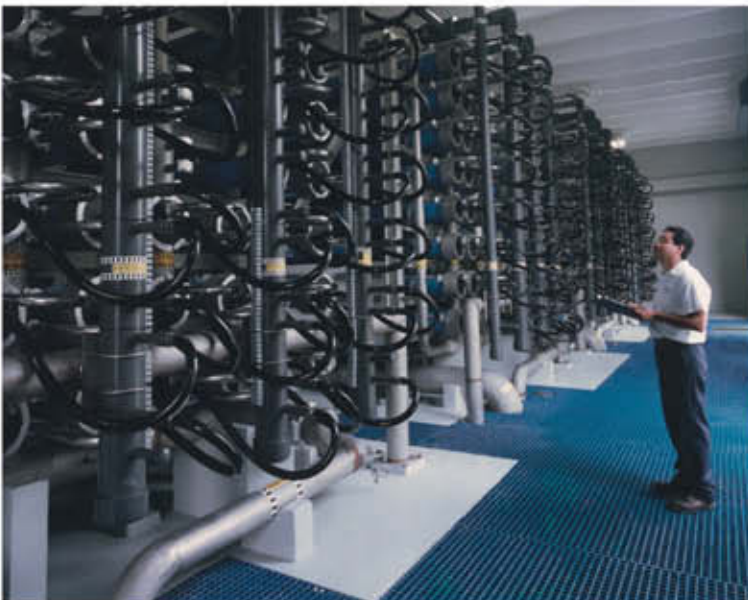
View of Reverse Osmosis installation
