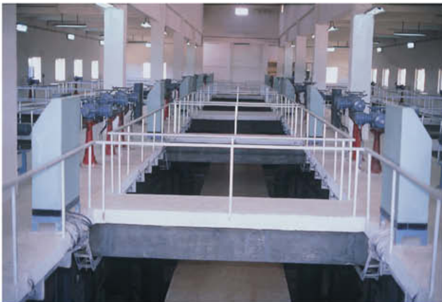
Filter house at a community water treatment plant
