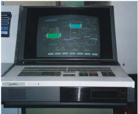
..... Insert of DCS Control System for Incinerator Plant
