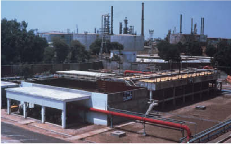
Partial View of Integrated 3 Stage Waste Water Treatment Plant for Refinery (1500 m 3 /hr)
