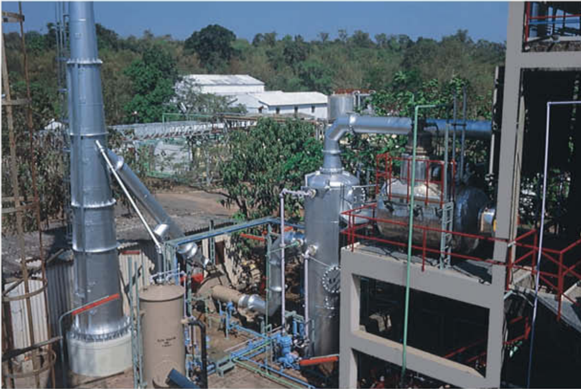
Incinerator Scrubbing System for a liquid waste incinerator
