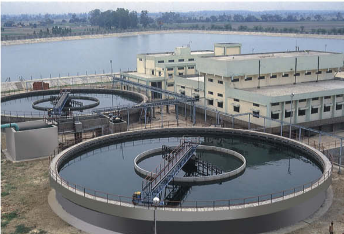
Bird's eye view - Water treatment plant at a Refinery
