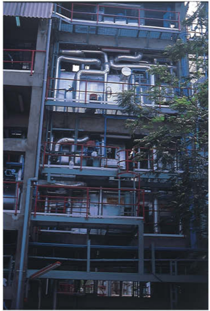
..... View of Waste Heat Recovery Boiler
