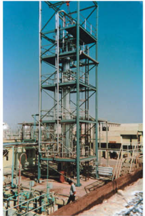
Wet air oxidation plant for Sulfide treatment at Gas processing complex
