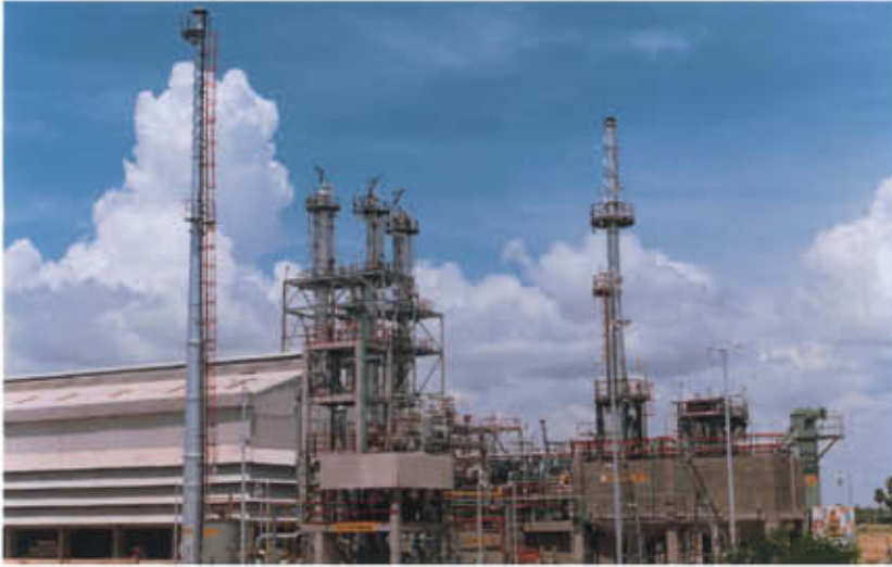
Acid Gas Incinerator at a Refinery
