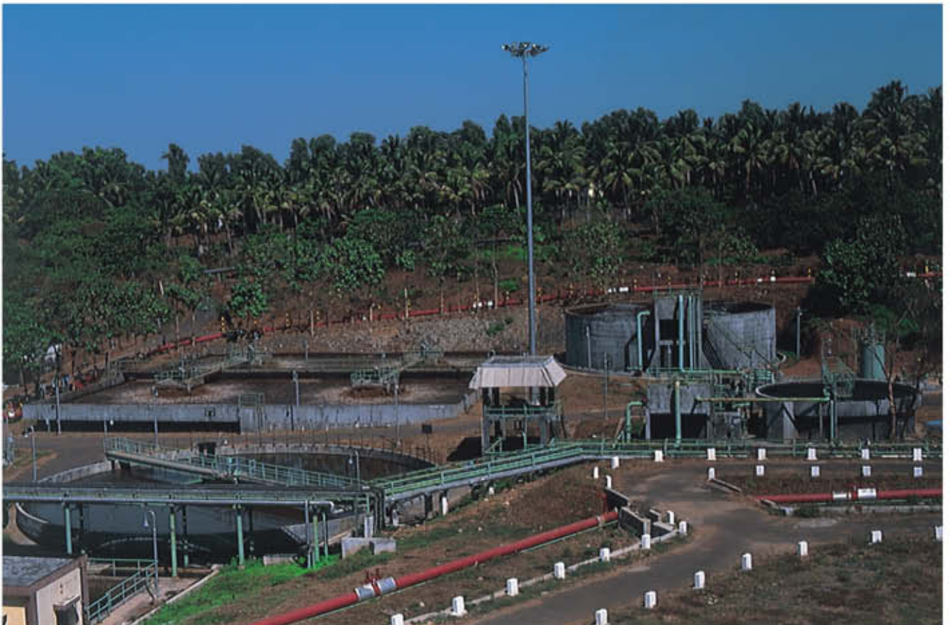
Effluent treatment plant at a 6 MMTPA Refinery Complex
