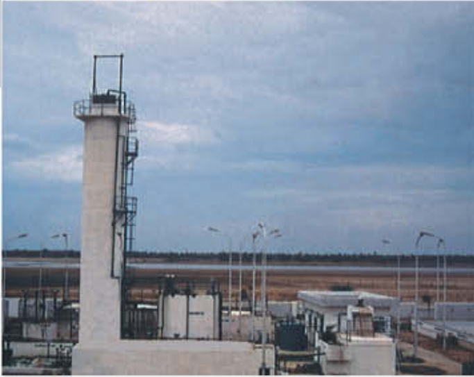
'Bio-bed' an anaerobic treatment facility for treatment of highly organic waste water for a Pharmaceutical plant
