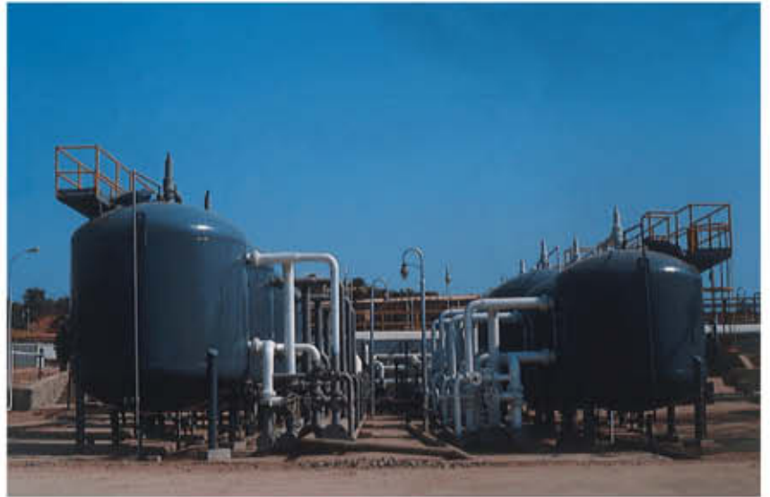
A battery of pressure filters as well as activated carbon filters
