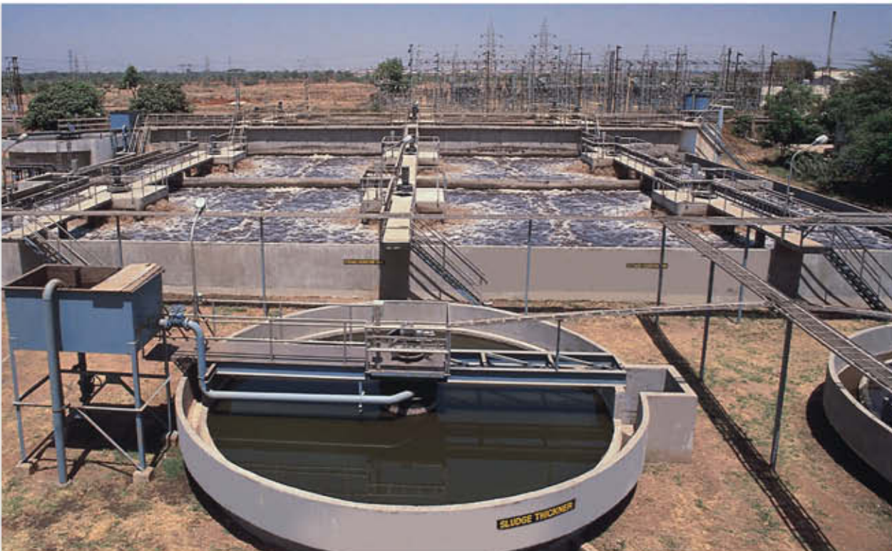
Effluent treatment plant for a Polymer Unit
