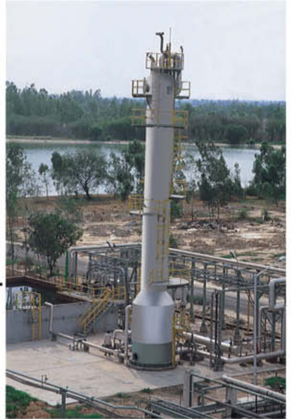
Ammonia steam strippers at a Fertilizer Complex
