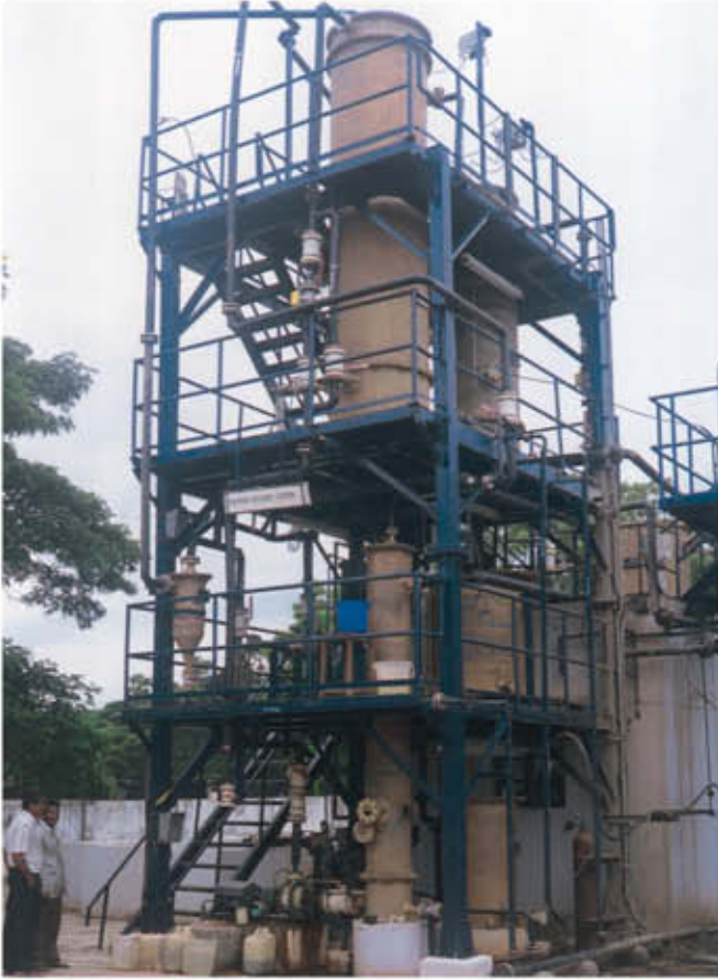
Sulphur recovery pilot plant for a Tannery unit
