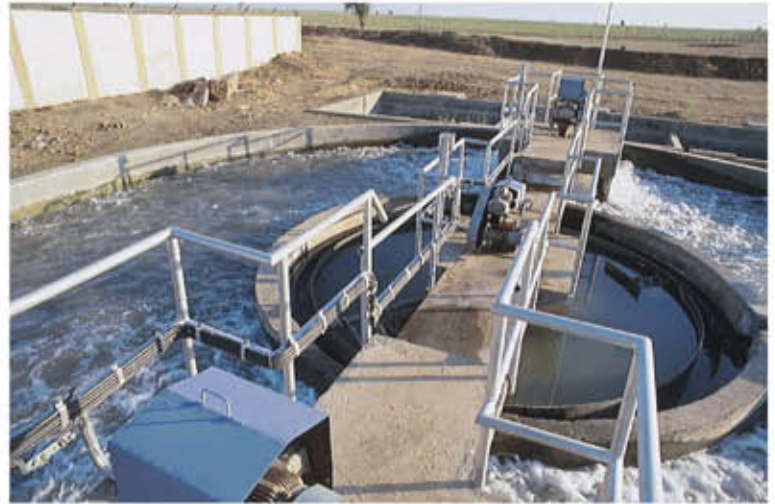
..... Package sewage treatment plant
