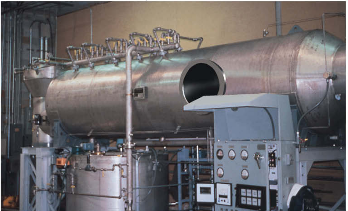
Packaged So2 Scrubbing System
