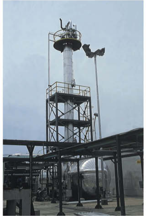
Ammonia Steam Stripper facility at a Fertilizer Complex
