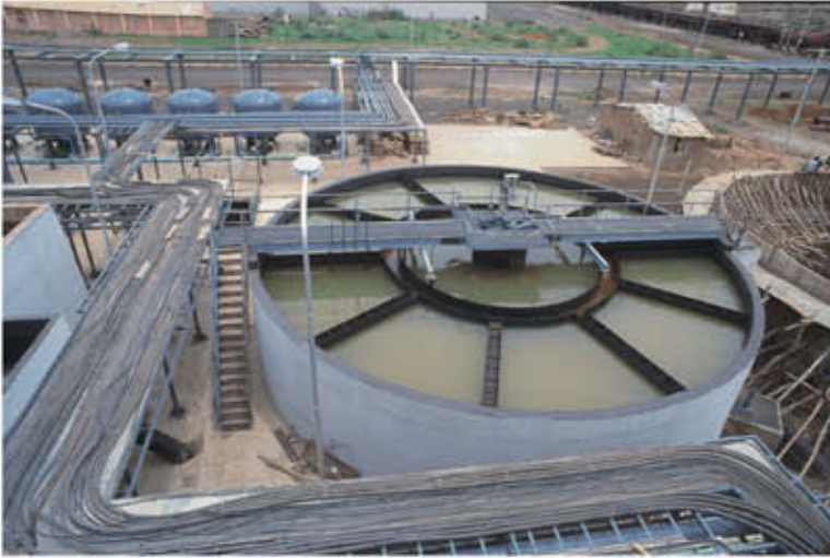
Reaction Clarifier for hardness removal at a Fertilizer Complex
