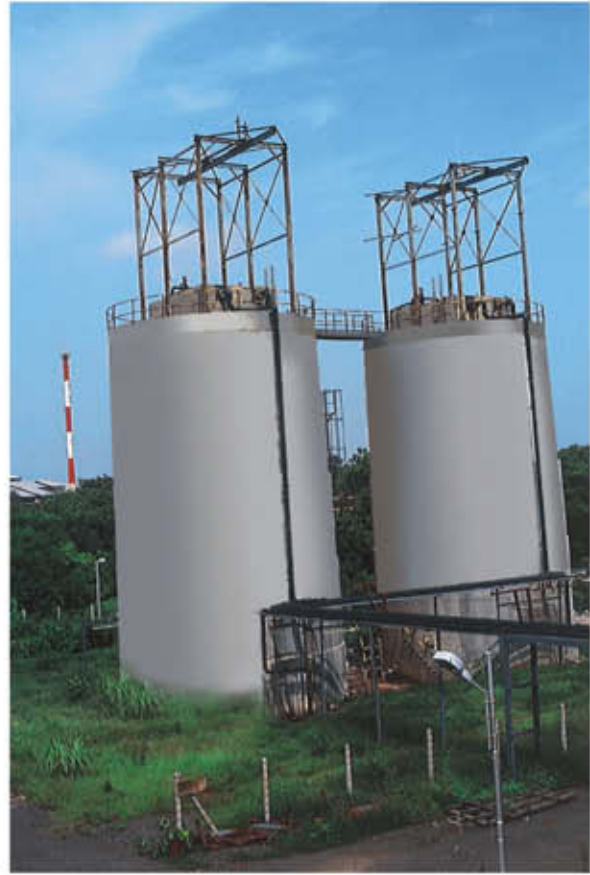
An integrated UASB effluent treatment facility for a Molasses distillery, Erythromycin & Penicillin Plant
