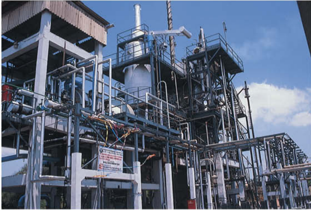
..... Rotary Kiln Incinerator at an integrated Petrochemicals Complex
